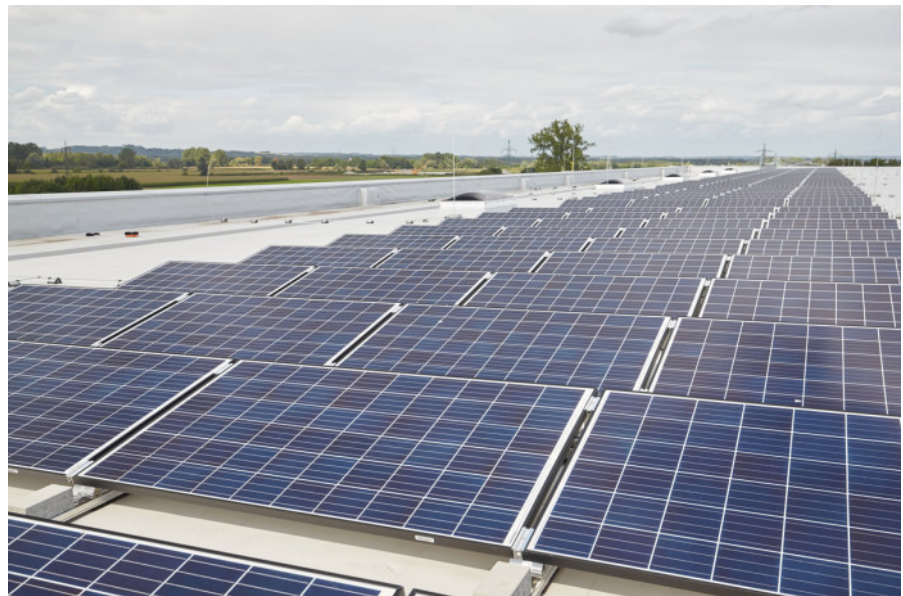
PV Anlage in Eitting, 2017
